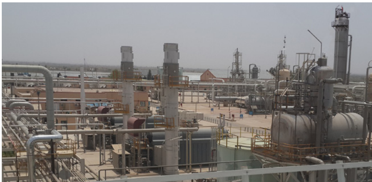
Uch gas processing plant, Dera Bugti, Balochistan.
