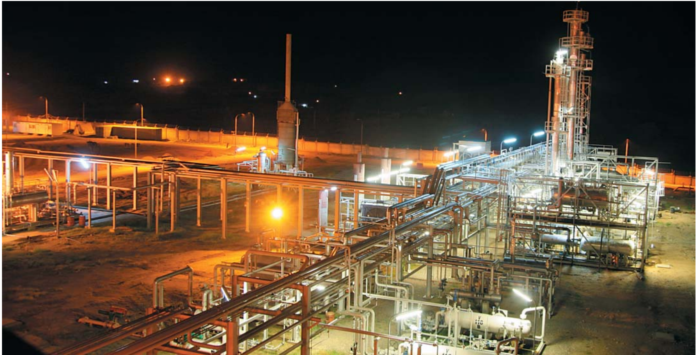
Chanda Gas Processing Plant
