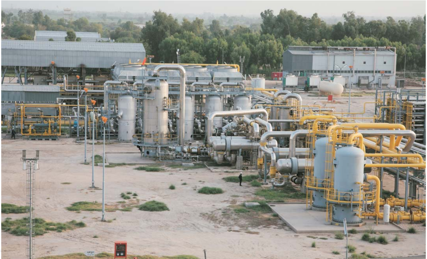
Qadirpur Gas Processing Plant
