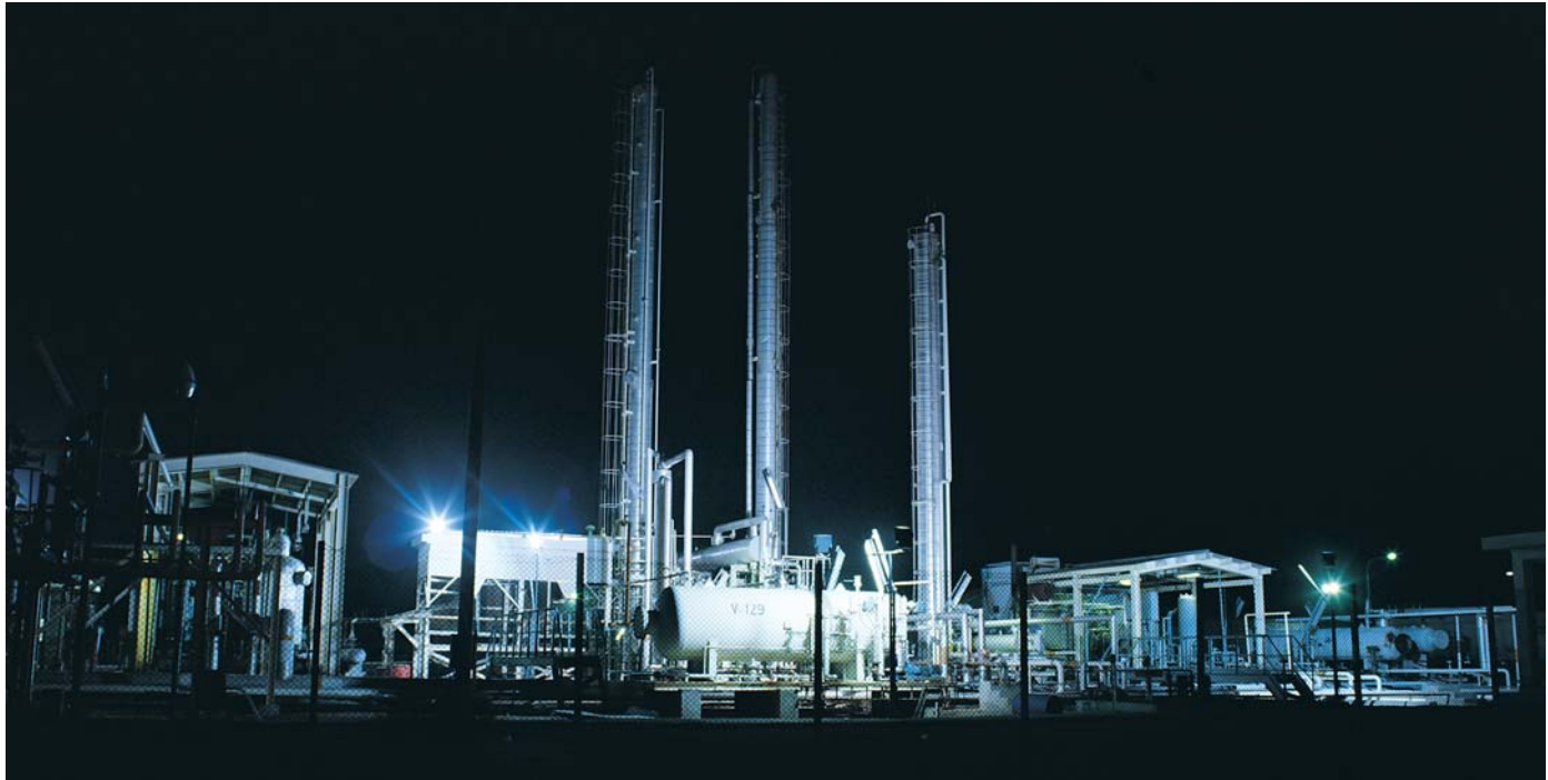
Kunnar LPG Plant
