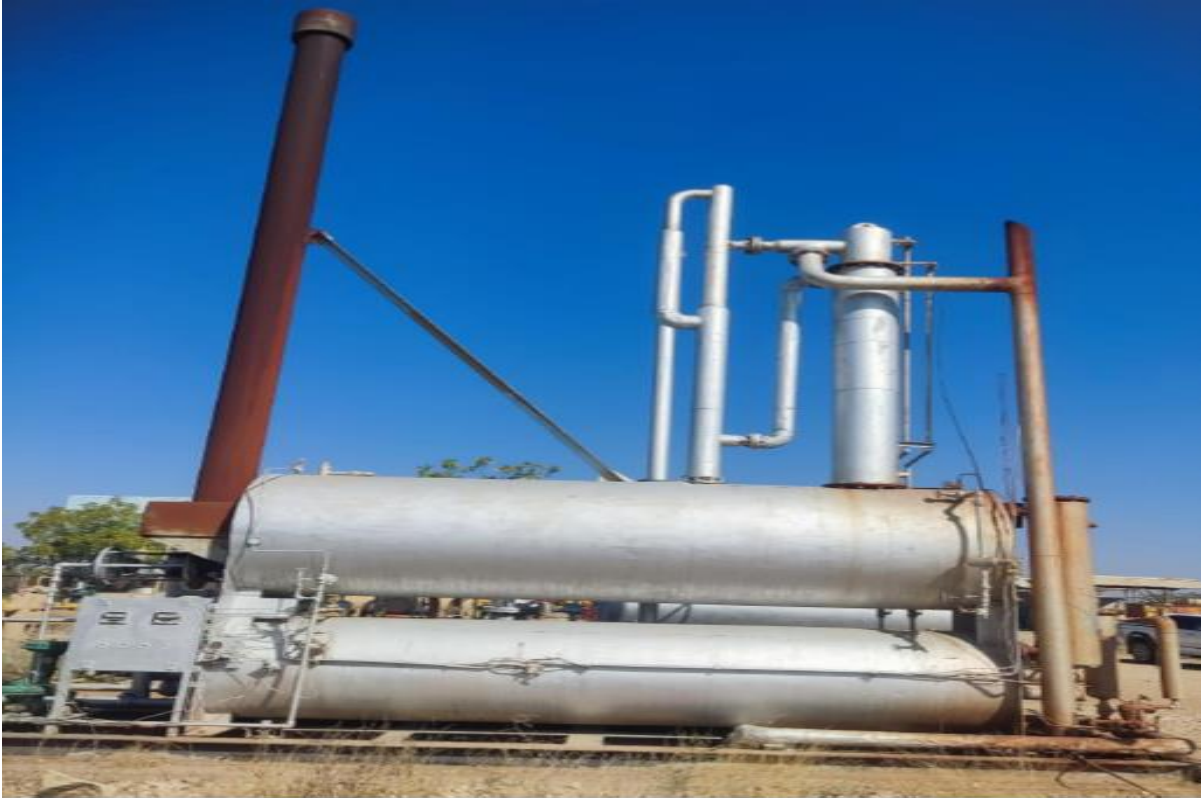
Figure (i): Glycol Re-boiler Skid
