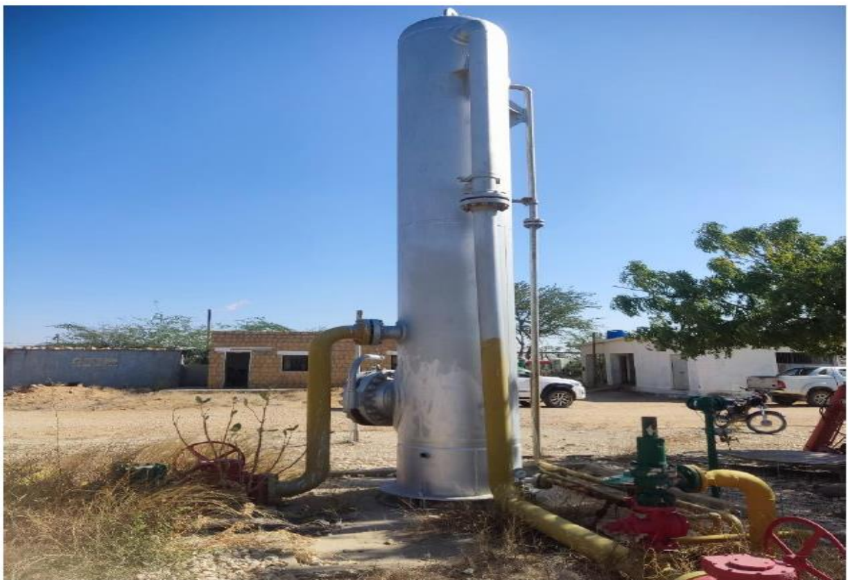
Figure (iv): Absorber Column Skid
