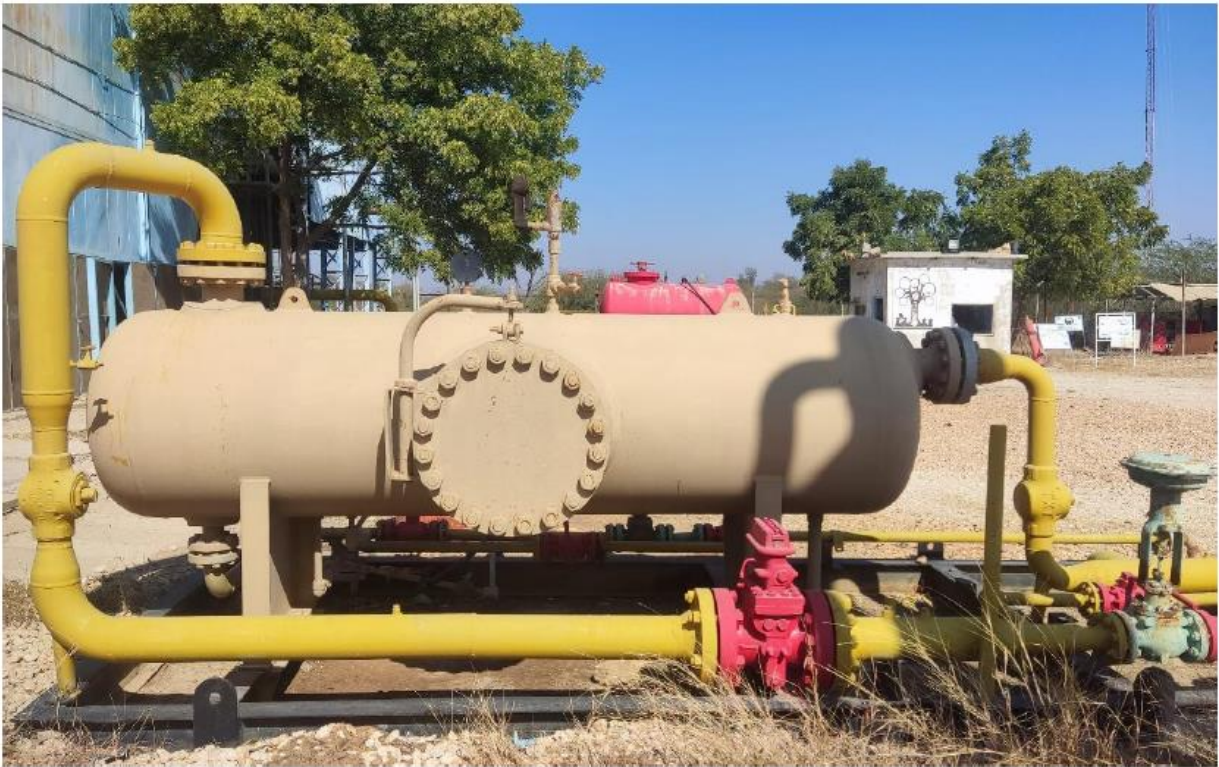
Figure (iii): Inlet Gas Separator Skid
