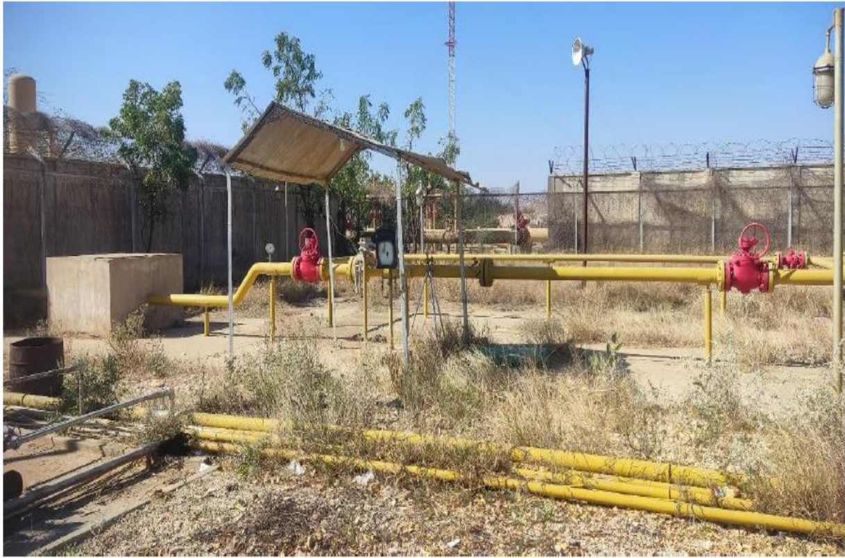
Figure (v): Gas Metering Unit
