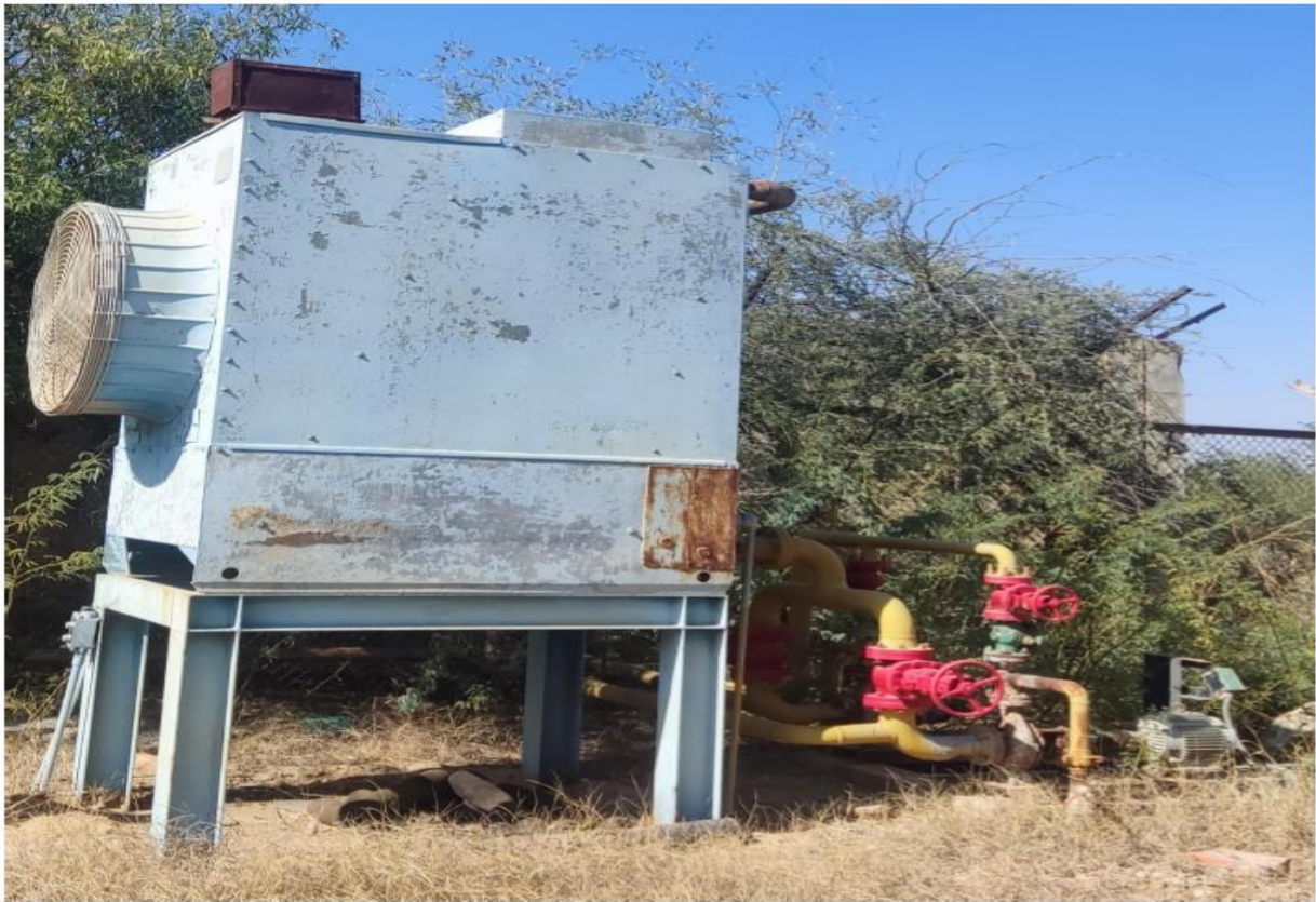
Figure (vi): Cooling Tower Unit along with Pumps
