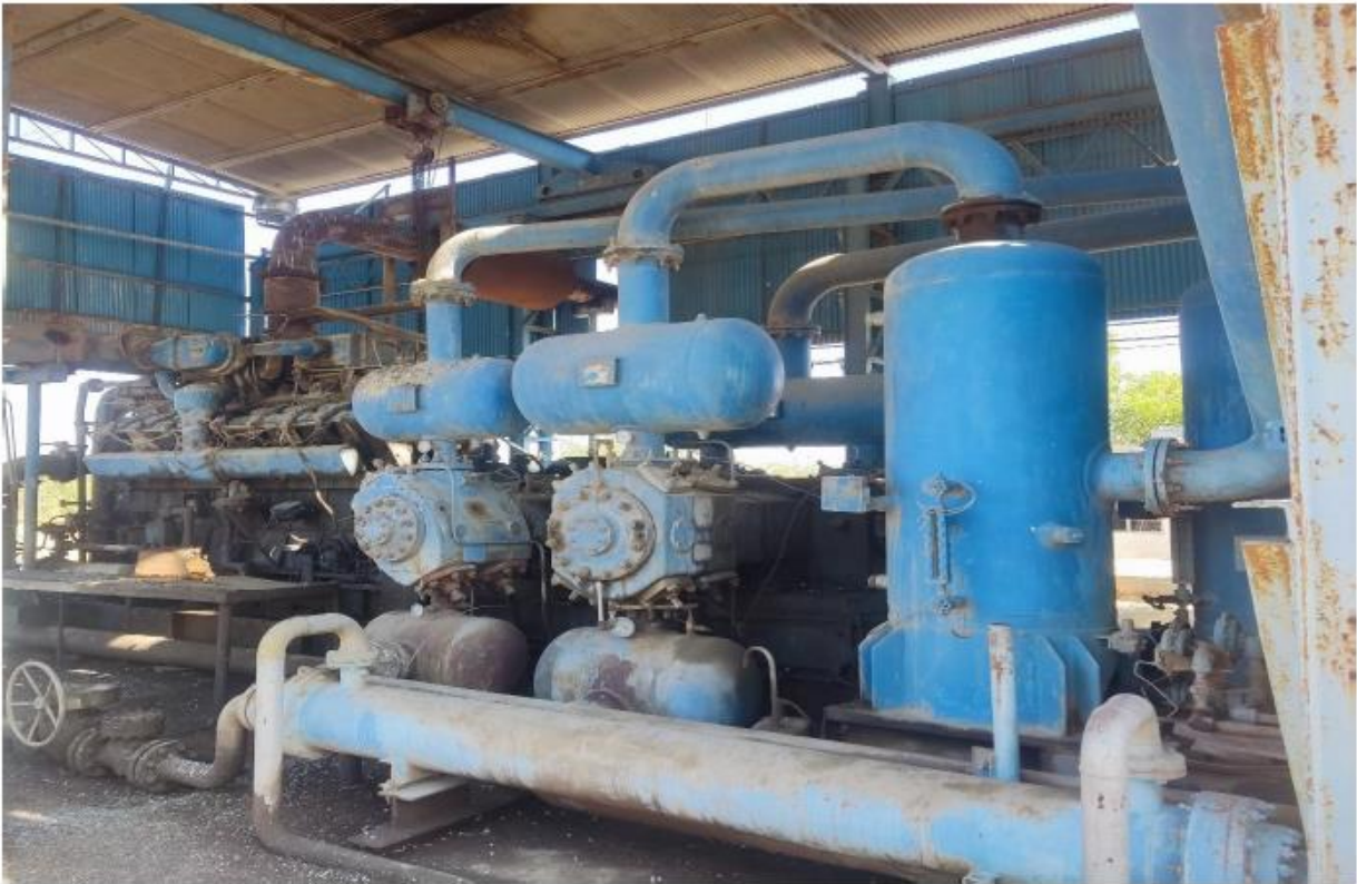
Figure (vii): Engine-Compressor Skid
