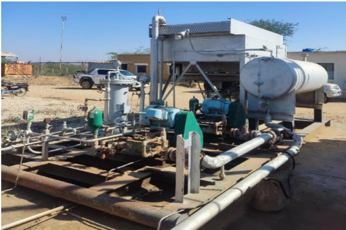
Figure (ii): Cooler & Pumps Skid
